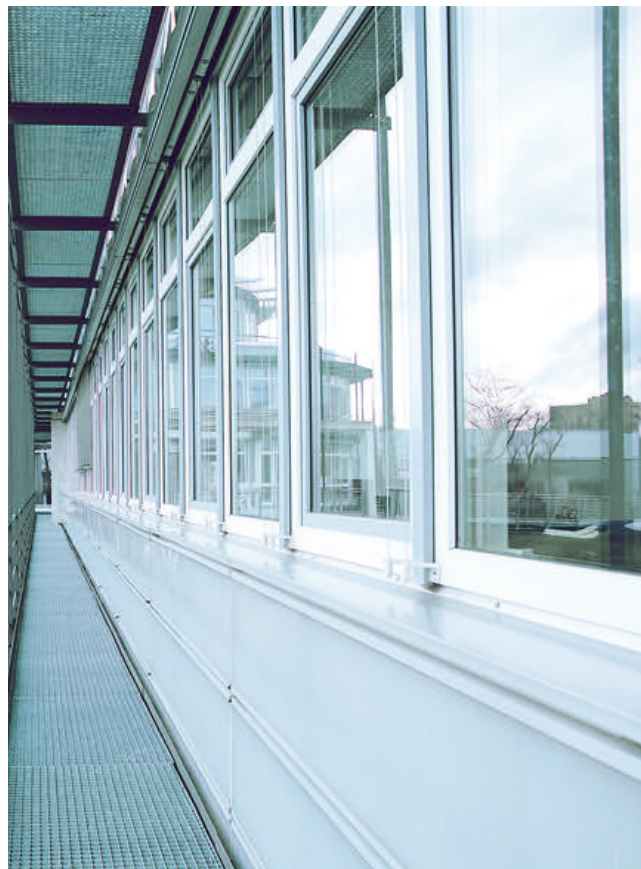
PVC windows are of course available in white, like the ones in this office building, but there are also other finishes, e.g. wood effect (photo: Baerlocher)
